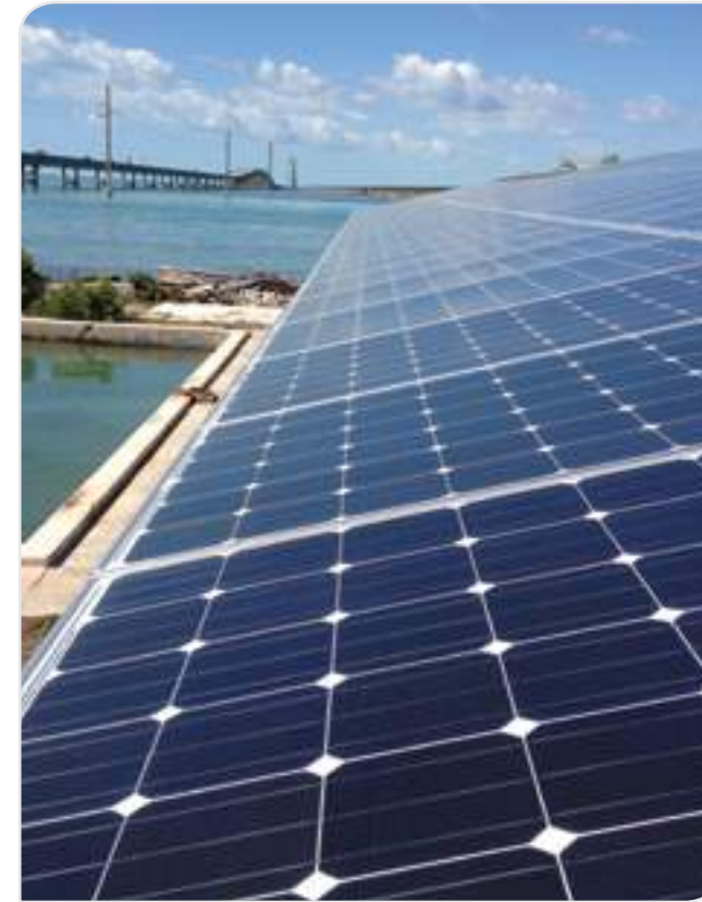
Florida, USA Off-grid solar 23 kW
