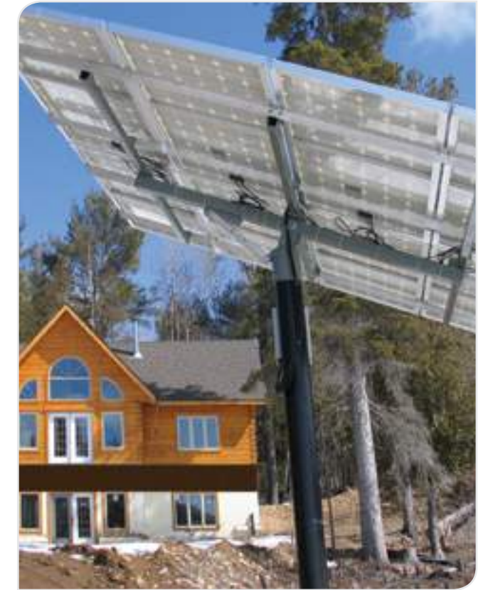
Ontario, Canada Off-grid solar 10 kW
