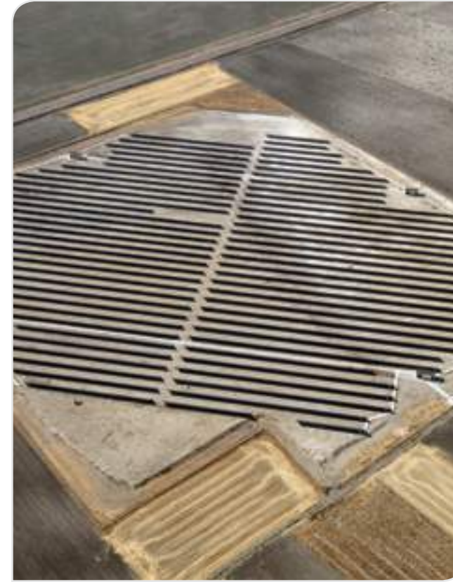
Villanueva del Aceral, Spain PV power plant 3 MW
