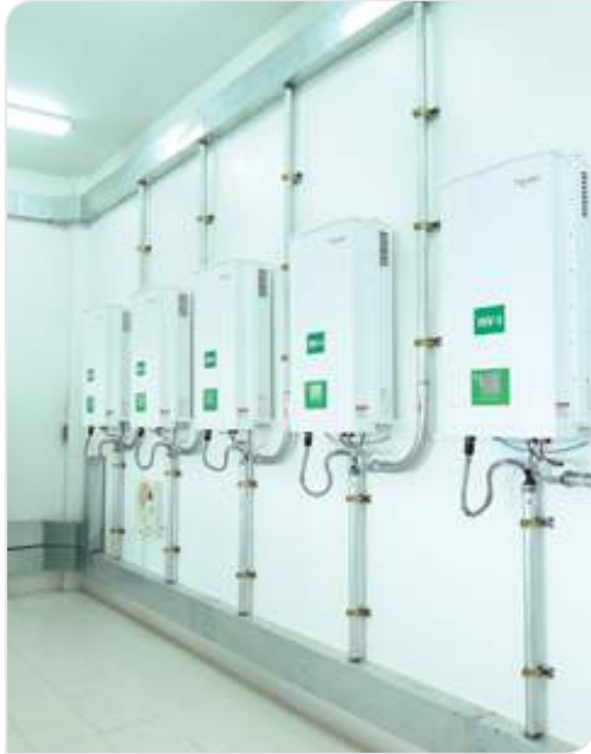
Phetchabun, Thailand PV power plant 3.3 MW
