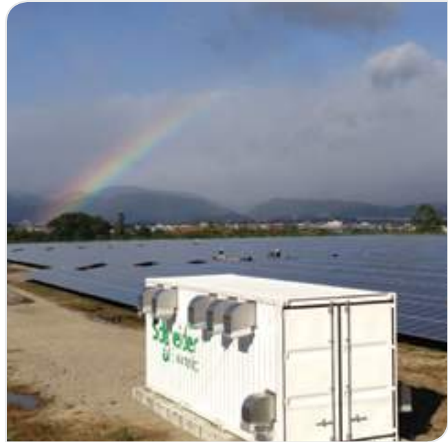
Fukusaki, Japan PV power plant 1.36 MW
