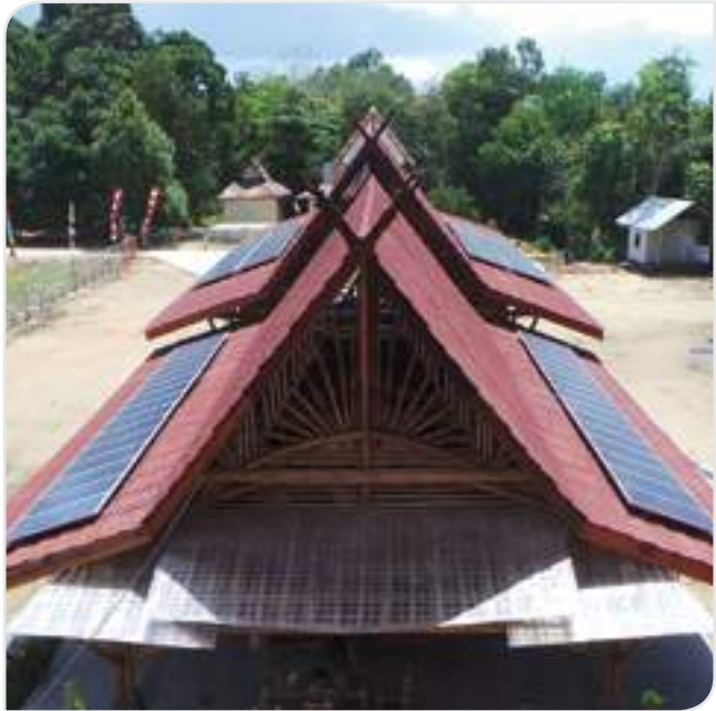
Borneo, Indonesia Off-grid solar 12 kW
