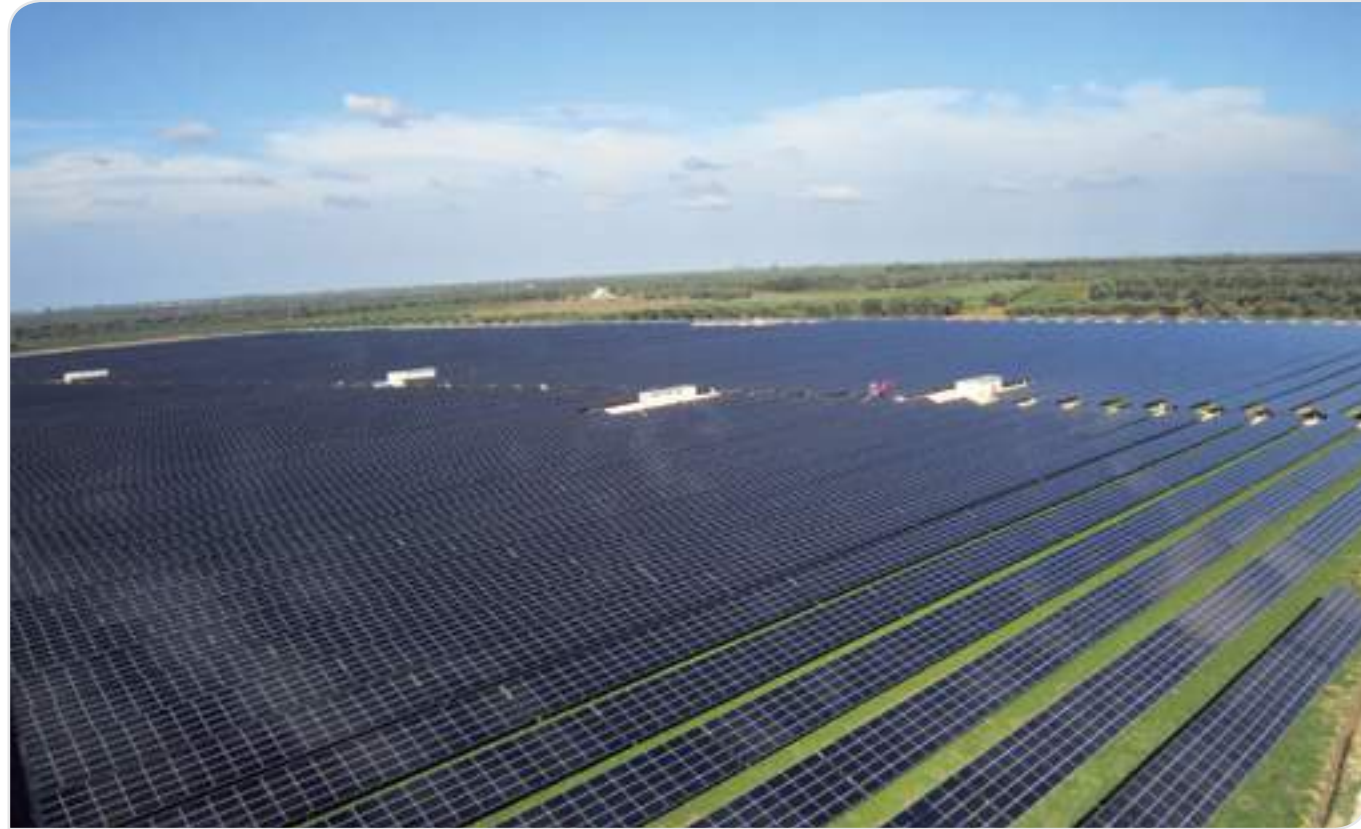
Plugia, Italy PV power plant 43 MW
