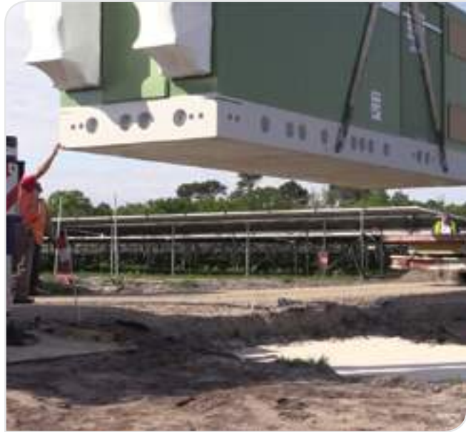
Cestas, France PV power plant 300 MW
