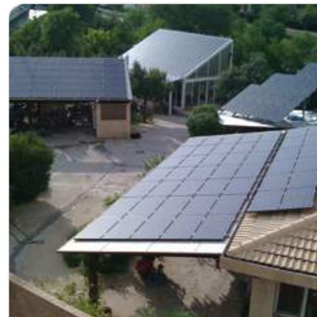
Madrid, Spain Off-grid solar 18 kW
