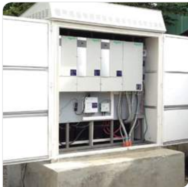
Philippines Telecom Towers 18 kW
