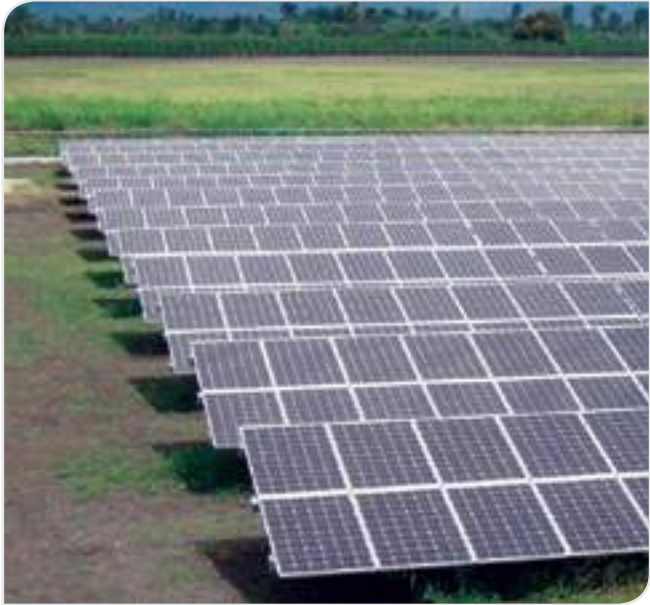
Cibao, Dominican Republic PV power plant 1.5 MW
