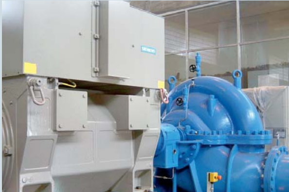
Variable-speed drives ensure profitable water supply in Madrid
