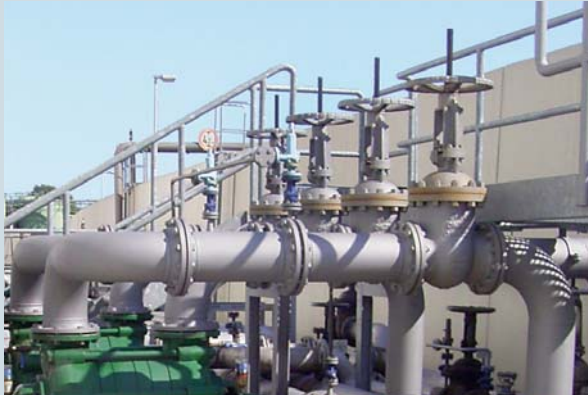
MICROMASTER frequency converter ensures cost-efficient diesel transportation at Shell
